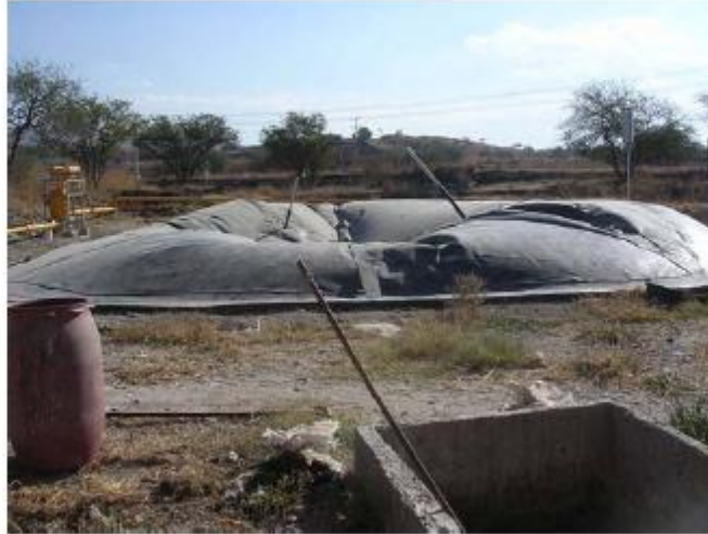
Collecting Tank and Anaerobic Digester. Farm Paraíso IV. Abasolo, Guanajuato. Mexico
